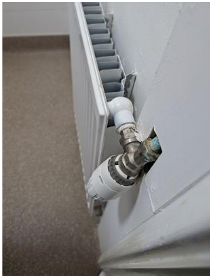
Radiator valve at waist height.
